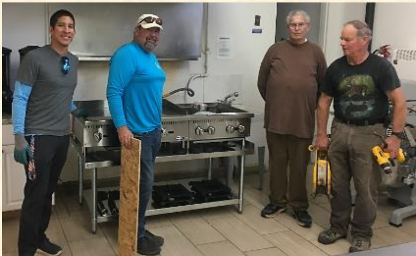
In With the New – L to R Lucho, Peter, Pat and Rick with the new cooking equipment installed.
